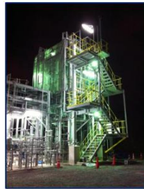
Pilot with commercial gasifier-run for 8 years
